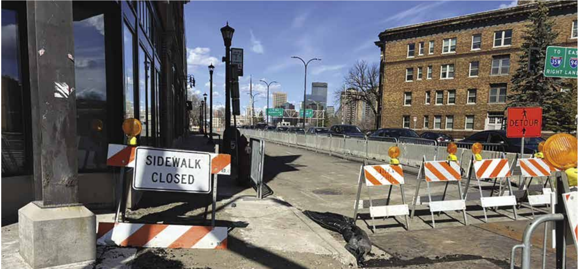
Traffic narrows along Hennepin Avenue in Minneapolis as crews carry out a major reconstruction project on a corridor that began as a Dakota trail connecting St. Anthony Falls to the city's lakes. The work is part of the city's effort to balance cars, buses, bikes and pedestrians on one of its busiest streets. (Image: Craig Wilson)
